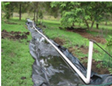
Larger beds can be built into the ground. Simply dig a trench line with plastic, lay in the distribution pipe, fill with organic material then back fill.
